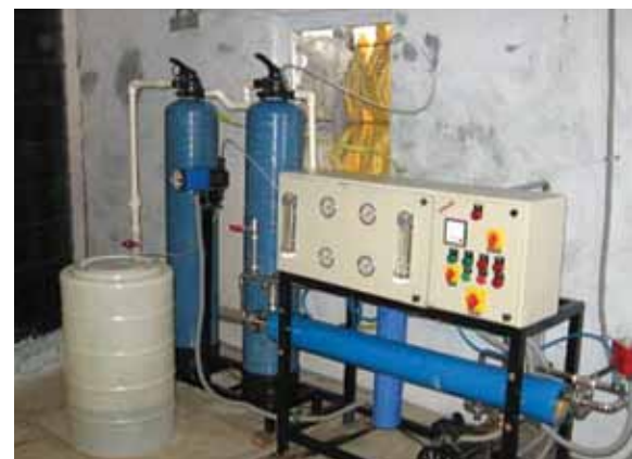
Machinery of water treatment plant.
